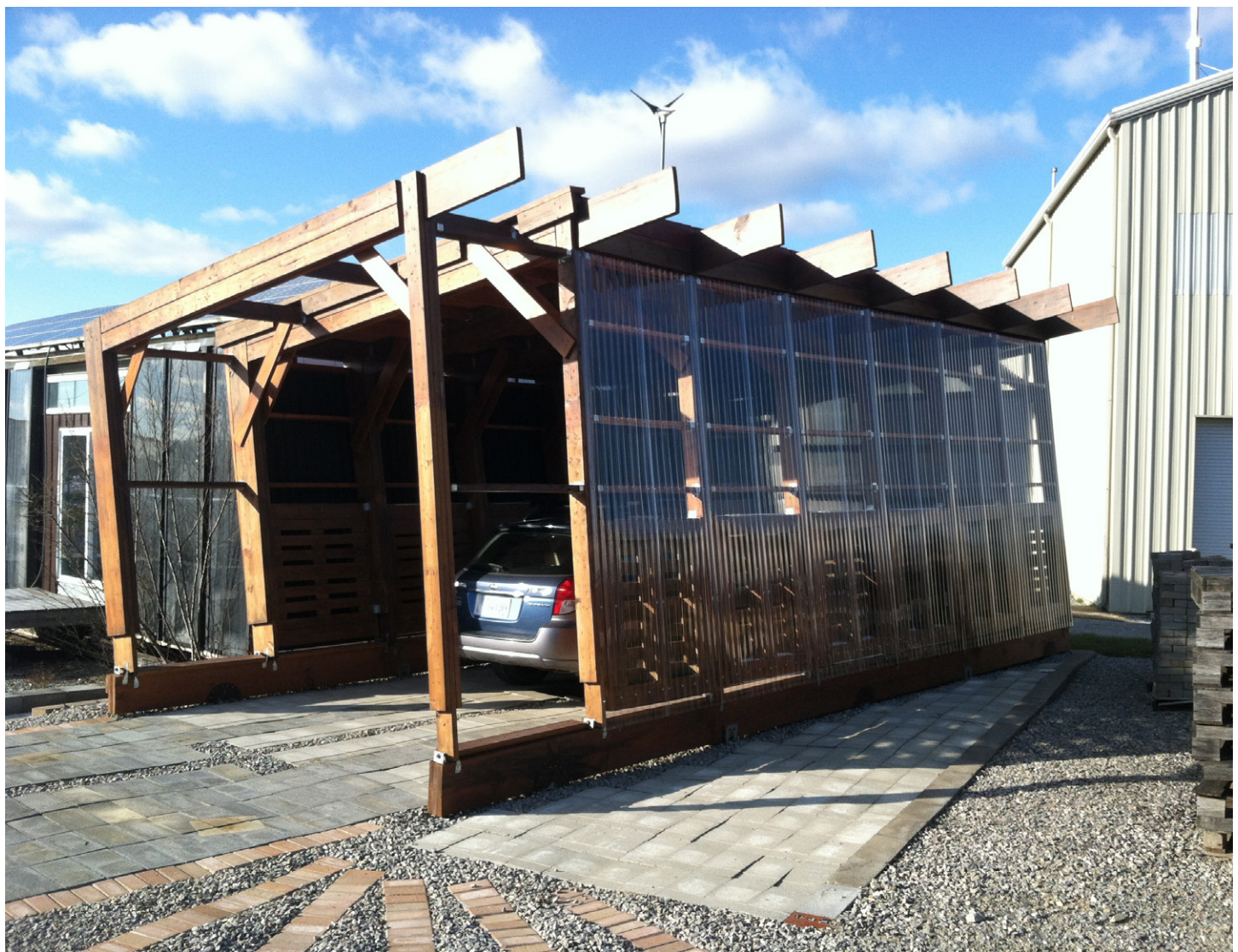
Full Scale Constructed works: Pallet Deck and Planter, Bus Stop, and Electric Car Garage 05 Design Frameworks
